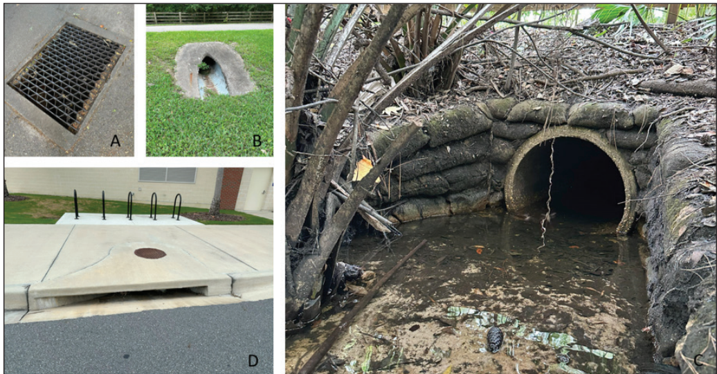
Figure 3. Example access points into the SSS of Alachua County. Stormwater grate in a road (A). Pipe openings at a body of water (B and C). Curb inlet on a roadside with a manhole (D). Photo credit: Alan Ivory, UF/IFAS
